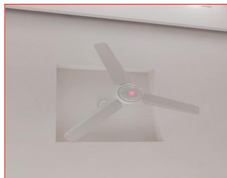
Fig 8: Photograph of BLDC ceiling fan
